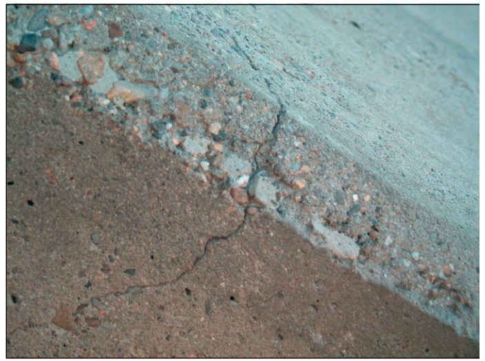
(b) Localized crack
