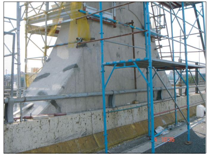
(d) Small local damage (segregation, small cracks) repairs with high adhesion cement mortar, added with polyvinilalcohol fibers
