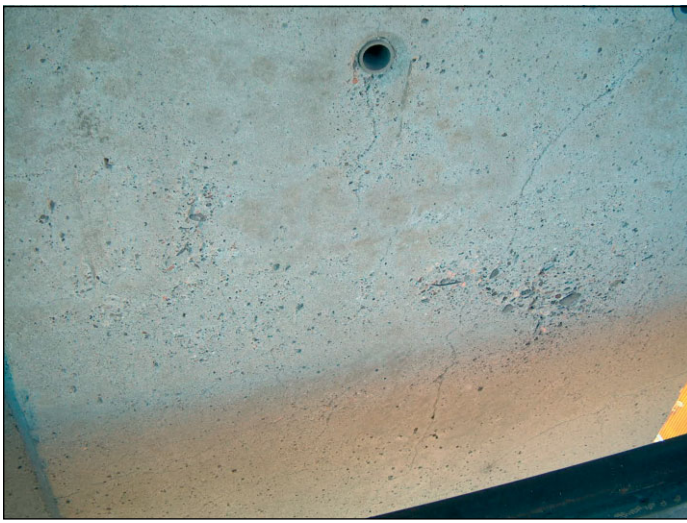
(a) Randomly distributed cracks
